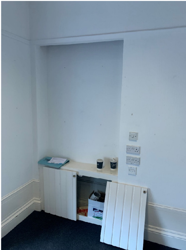
Ground floor linen press, with additional boxing in and face-plates. Additions to be removed and made good. Generous skirtings and picture rail to be maintained.
