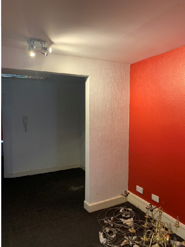
Later partition walls and lowered ceiling to the ground floor internal room to be removed, thus reinstating the form of the original drawing room. It is expected that the original ceiling and plaster cornice will be present and in a good or repairable state. If not then those to the front of the property will be used as templates for the recreation and reinstatement of the same.
