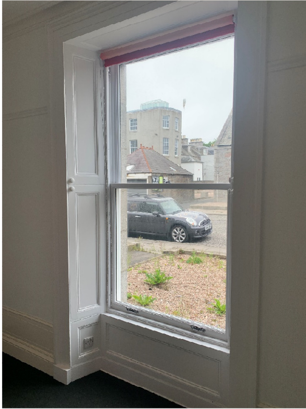
Ground floor window to Victoria Street; existing sliding sash casement window with timber panelled ingoes – original shutters – and moulded architrave and skirting. All to be retained.
